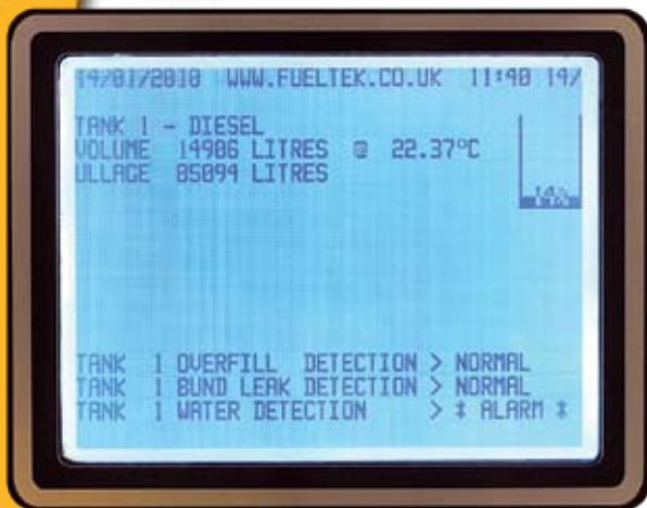
INFORMATION DISPLAYED AT THE FUEL TANK
